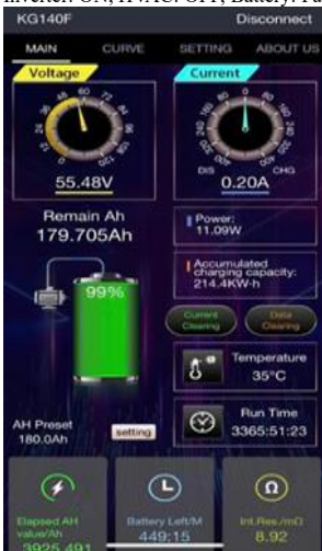
Scenario 2: Power Source: OFF, Inverter: OFF, HVAC: OFF, Battery: Full
